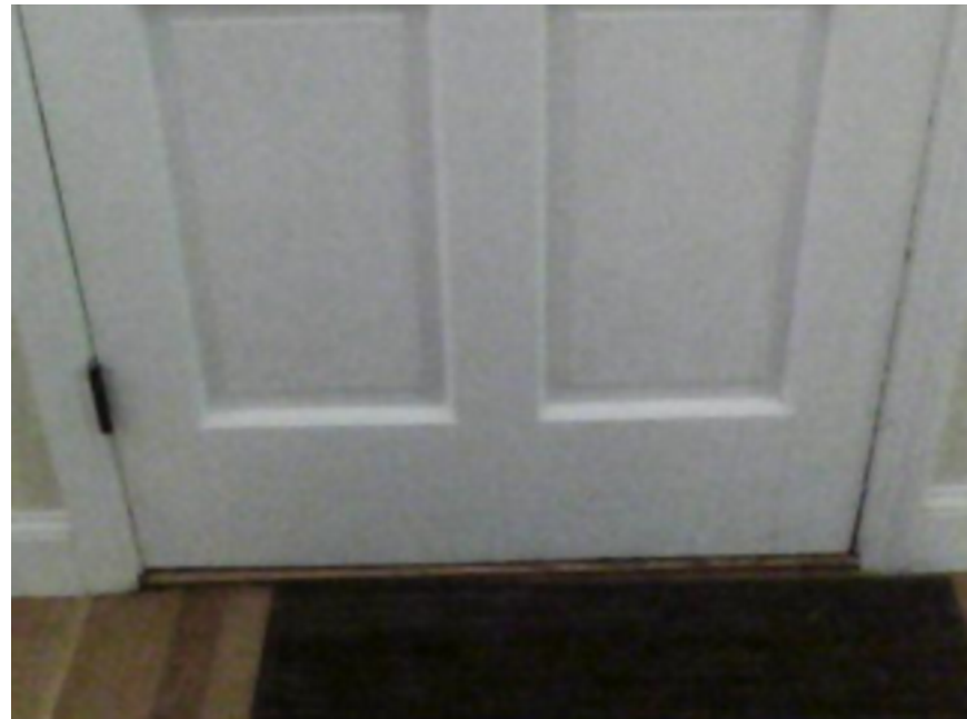
Cold air exfiltrating from in... FLIR E8 63900288
